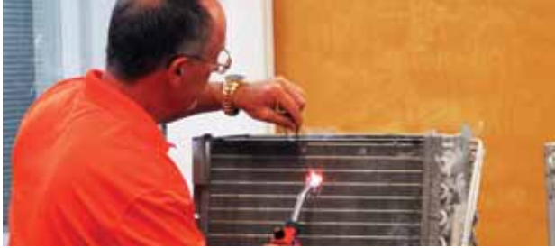
Gil Ledoux of PED Associates demonstrates how to repair an aluminum coil leak that is within the fin section.
