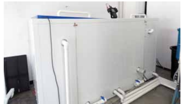
500 gallon rinse and chemical tanks were installed to filter and reclaim the pre-treatment chemicals to be reused again and again
