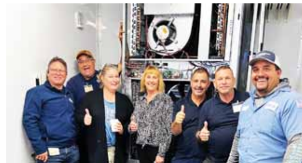
Employees of the Hillsborough County Public Schools attended an I-TEC presentation of the Bard stand alone vertical package unit
