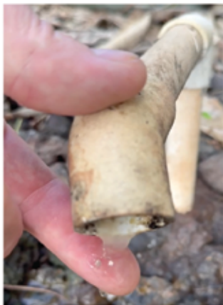
HVAC condensate completely laden with Zoogloea
