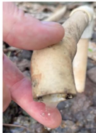
HVAC condensate completely laden with Zoogloea
